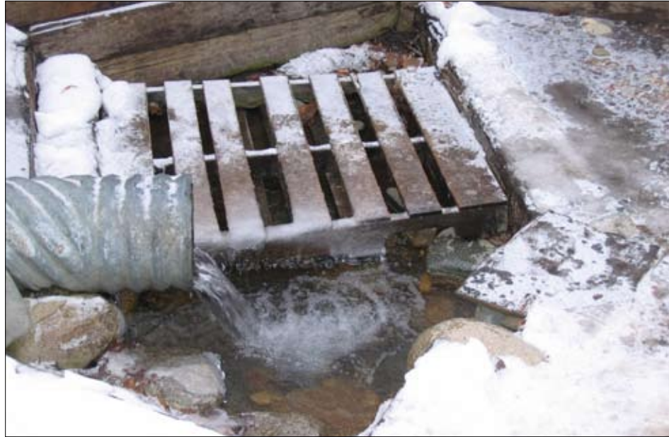
This outfall contains fresh spring water, according to those who have used it for decades. The state calls the water road runoff. The Borough may eventually settle the matter by hiring a hydrologist.
